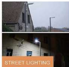
BLACK SPOTS LIGHTING
